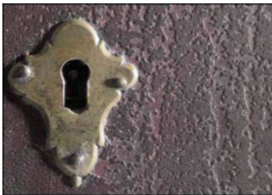
Figure 4. Detail of degraded door finish.
